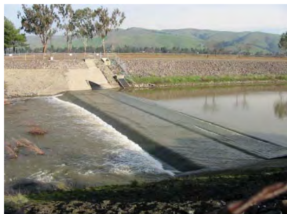
Alameda Creek rubber dam in the “down” position
